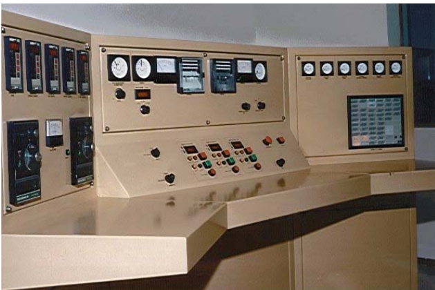
Figure 4. The IPR-R1 Reactor New Control Console
